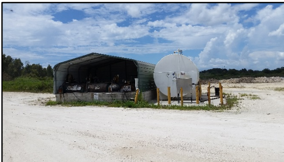
F) Chemical tank well and storage tanks
